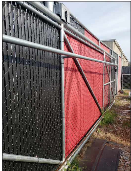
Long gates also need lateral trussing to resist wind and the tendency to “lean over” to one side. Often referred to as a “strong arm” support, this is a 1 ft wide “panel” attached perpendicular to the gate, running the full length of the gate. This is especially important for privacy style gates, or any gate with significant infill to catch the wind.
