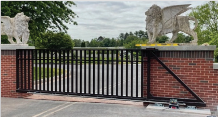
Typical: Diagonal trussing in the vertical dimension is needed for all gates. A simple diagonal in the tail section will work for many “smaller” gates.
