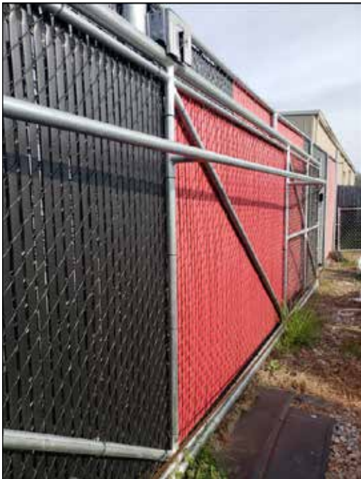
Long gates also need lateral trussing to resist wind and the tendency to "lean over" to one side. Often referred to as a "strong arm" support, this is a 1 ft wide "panel" attached perpendicular to the gate, running the full length of the gate. This is especially important for privacy style gates, or any gate with significant infill to catch the wind.
